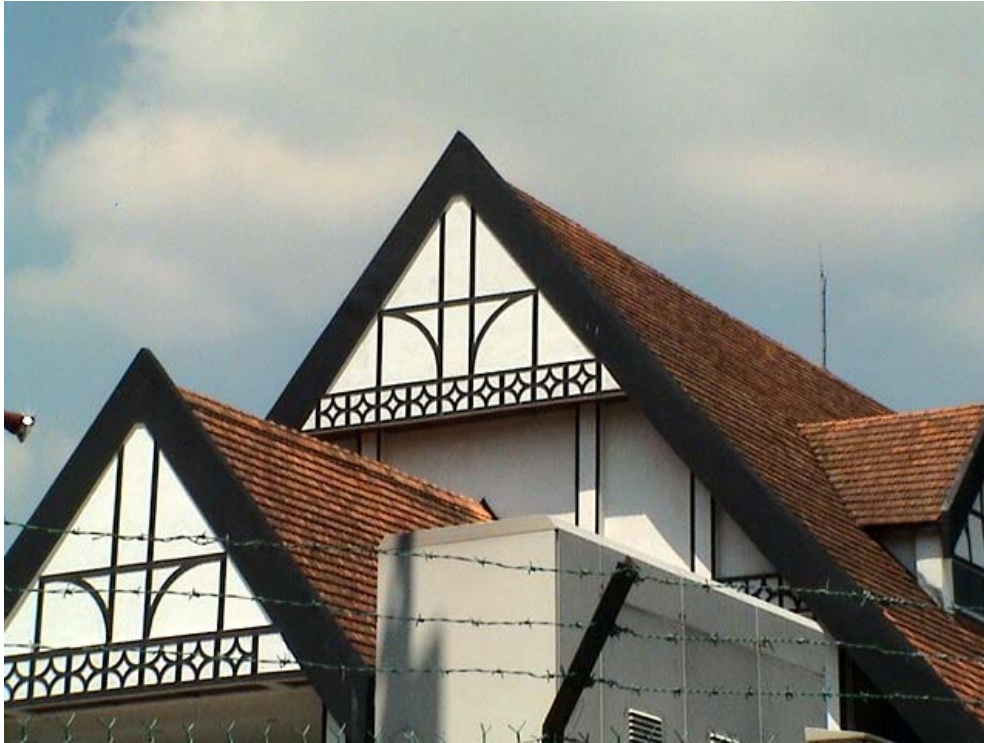
Figure 10: The repaired façade and the new Spanish made ESE air terminal in 2004.
