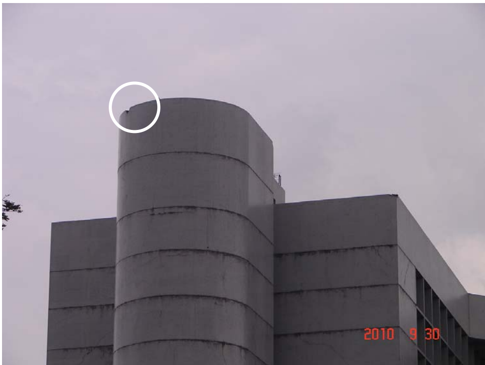
Figure 16: A bypass on the curved edge of the parapet wall on the west wing of the DCS building.
