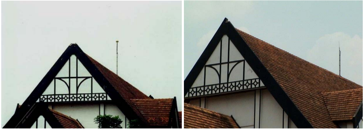
Figure 12: The bypasses at the RSC building suggest that neither the CVM nor the ESE standard, NF C 17-102, is a valid air terminal placement method.
