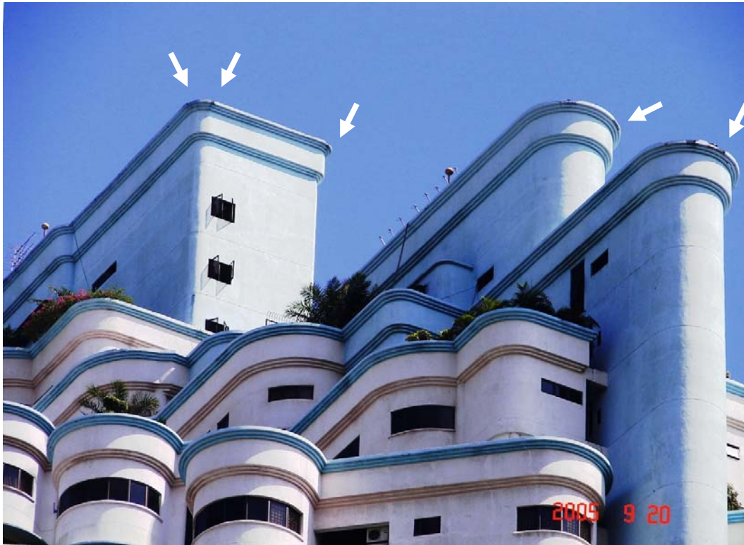
Figure 19: Five additional bypass locations were observed on the edges of the upper, middle and lower curved roofs in 2005.
