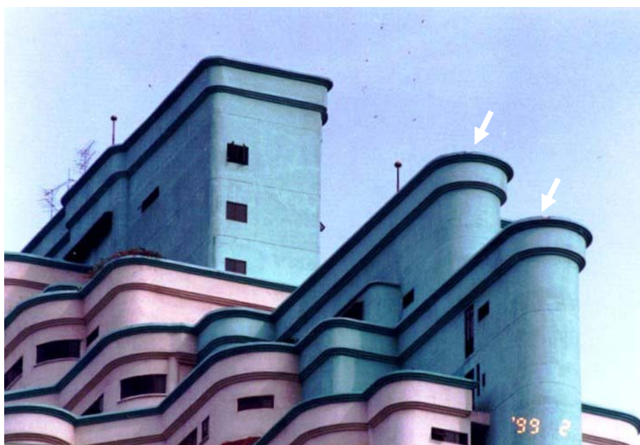
Figure 18: Two bypasses observed on the edges of the middle and lower curved roofs in 1999.
