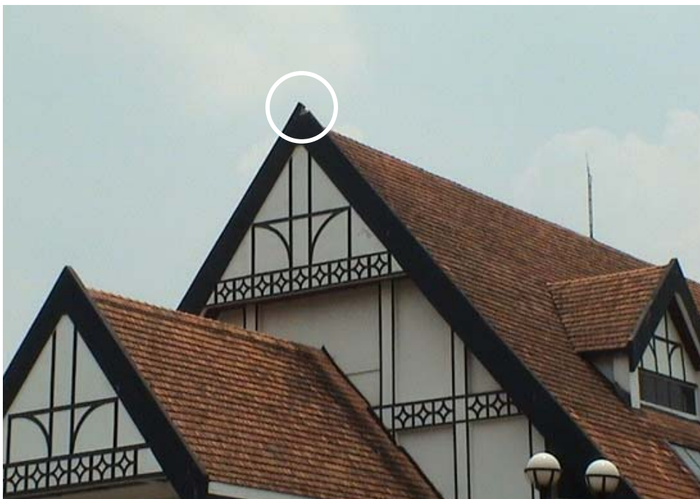
Figure 11: In 2005, another bypass was observed at the same front facade.
